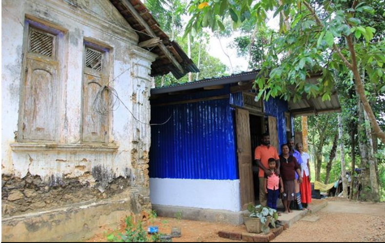
Mr. Gihan Nilanka and his family from Kalutara District outside their transitional shelter. Their flood damaged house is in the foreground.
