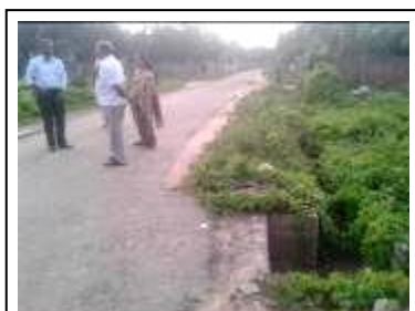
A view of built road drain, which is effective but not being well maintained
