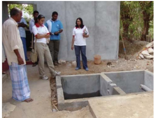
Technical officers from the District office inspecting the construction of a sewerage tank
