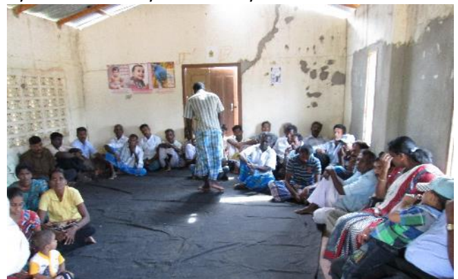
The interior of the damaged community centre
