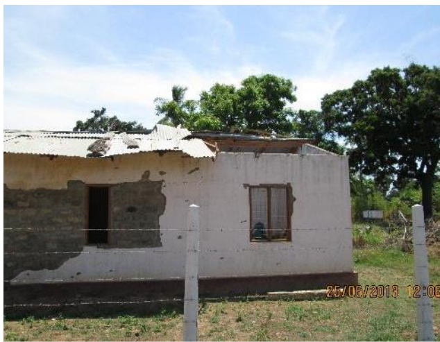
The damaged community centre in Thiruvaiyaru
