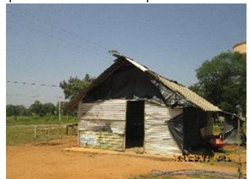
Damaged preschool at Sivanagar
