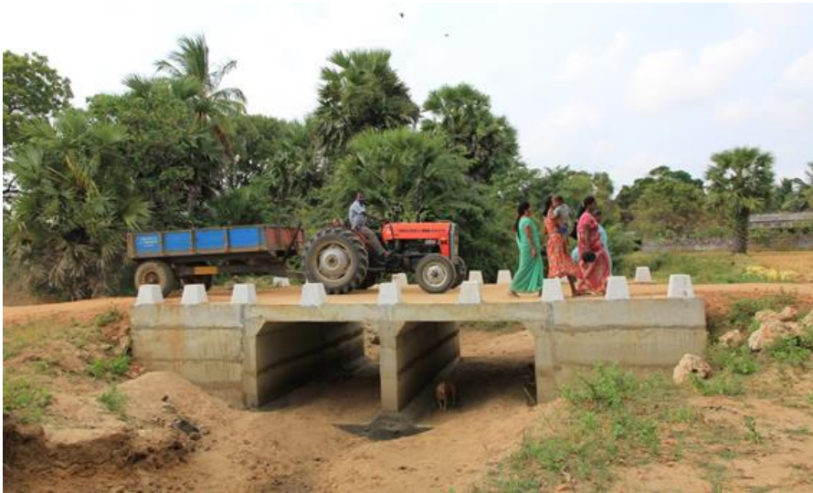
The SWD structure which doubles up as a small bridge is regularly used by pedestrian and vehicular traffic.
